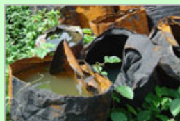
Open tar drums at road construction sites.
